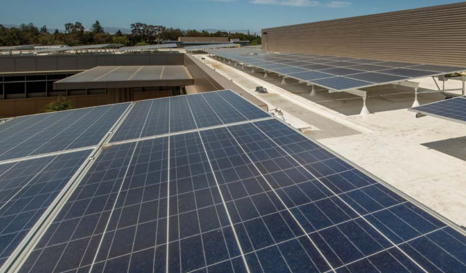
Solar panels on the roof of net zero energy Hanover Page Mill office building in Palo Alto, CA.
