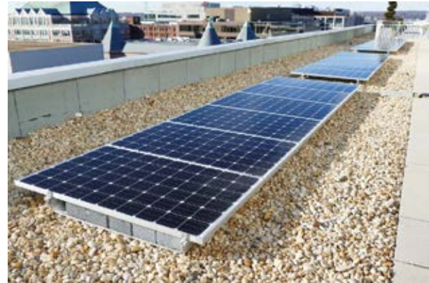
The Millennium building's rooftop PV. Credit: The Tower Companies
