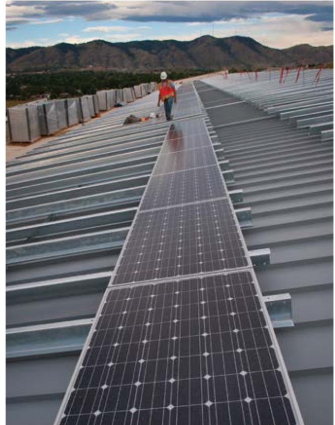
Credit: Dennis Schroeder / NREL
